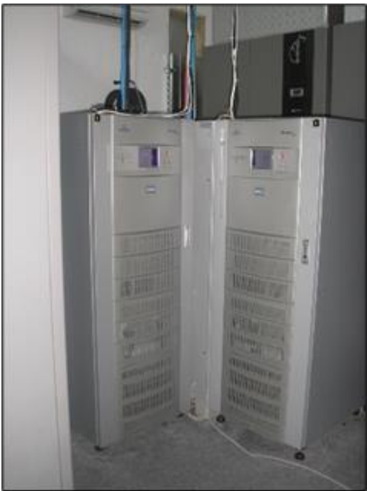
UPS Emerson Liebert
